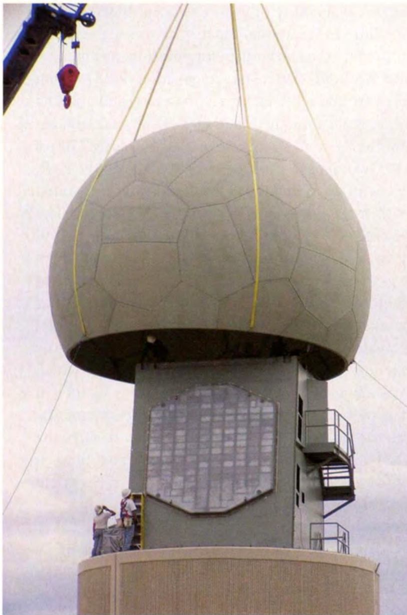
FIG. 4. The NWRT: Installation of the radome over the single aperture of the AN/SPY-1A radar antenna.
